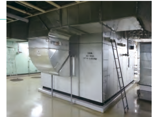
Air conditioning system for Hall B
